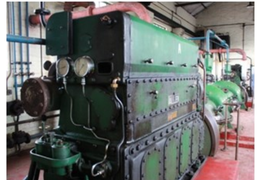
Diesel Engine driving the old pumps
