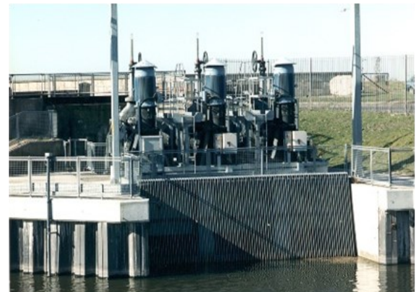
Crossens Pumping Station in the early 1990's
