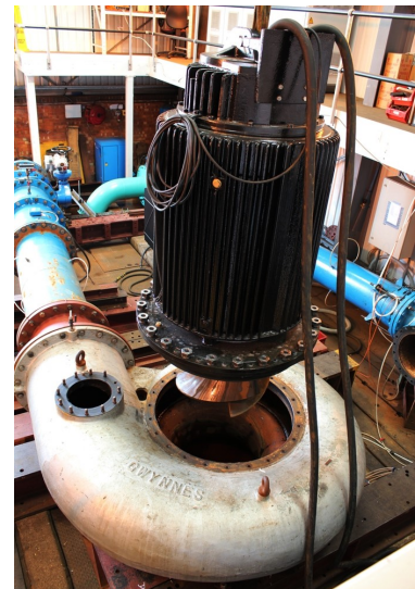
Fig 2. Bedford Pumps new rotating element utilises the existing pump casing
