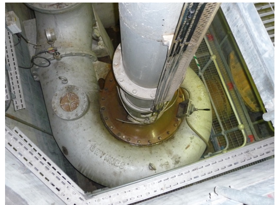
Fig 1. Existing Allen Gwynne pump installed at Netheridge
